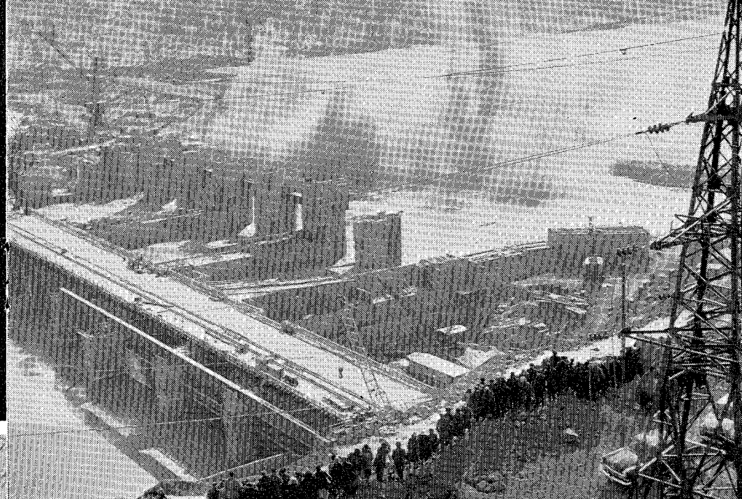
Above: Dynamiting the coffer-dam during the building of the Krasnoyarsk Hydro-electric Station on the River Yenisei. When completed this will be the biggest in the world.
